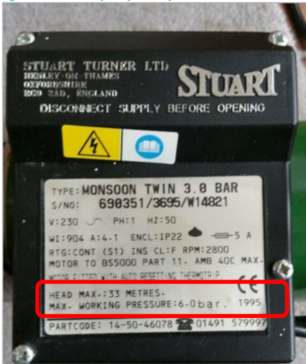
Figure 8.18 - The pump data plate – Maximum Pressure is 6 bar.
