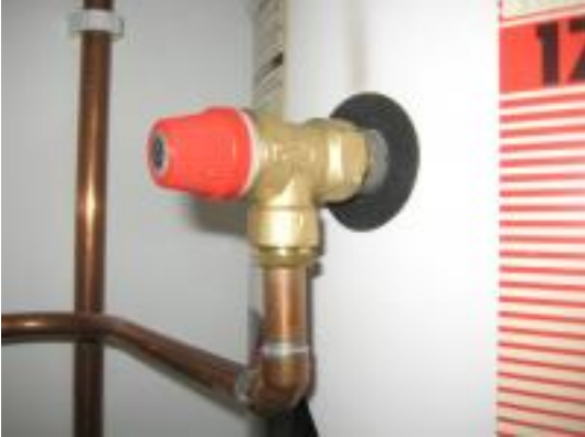
Figure 8.7 – A Relief Valve installed on a hot water cylinder.
