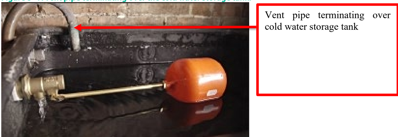
Figure 3 - A vent pipe terminating over the cold water storage tank.
