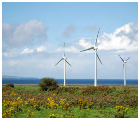
4.8MW Wind Farm
