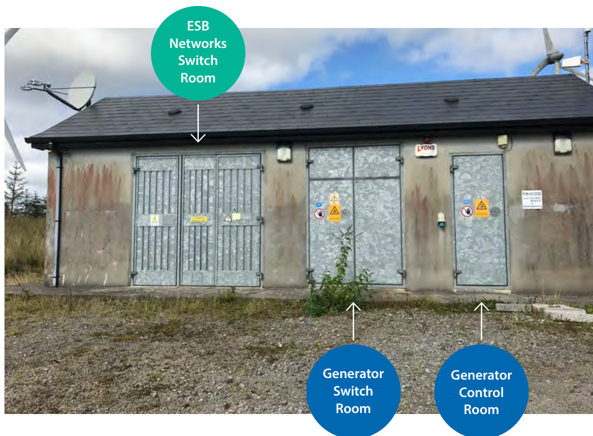
Figure 7: On Site MV Substation
