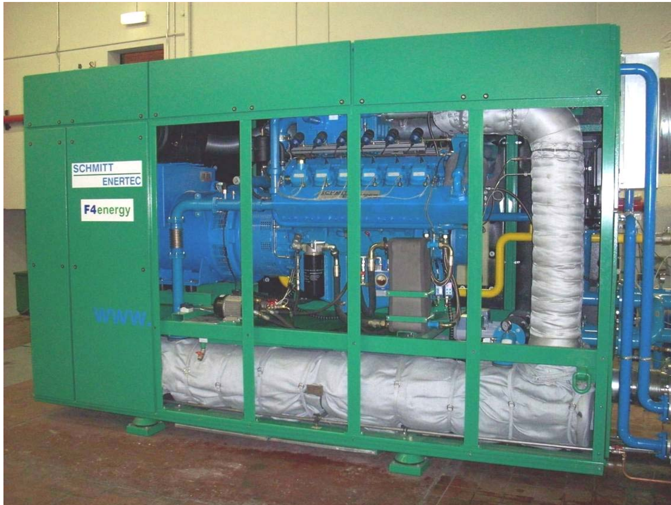
Plant Footprint: 4 meters Long X 1.45 meters Wide X 2.45m High
