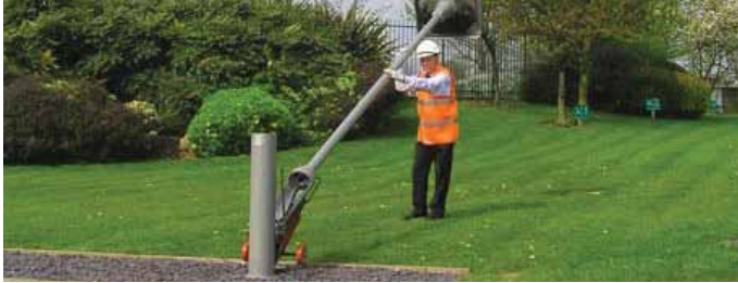
Fig. 6 The bottom-hinged column requires a bespoke tool, but with smaller columns is easily maintained by a single person
