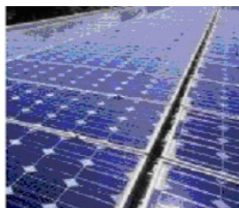
Close up of solar panel
