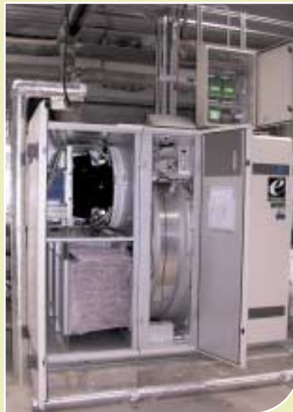
An internal view of the new AHU, including extract air fan, thermal wheel, air inlet filters, and cyclon control panel
