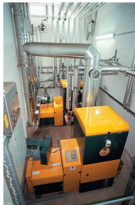
Wood pellet boiler
