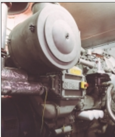
Inside of CHP Enclosure
