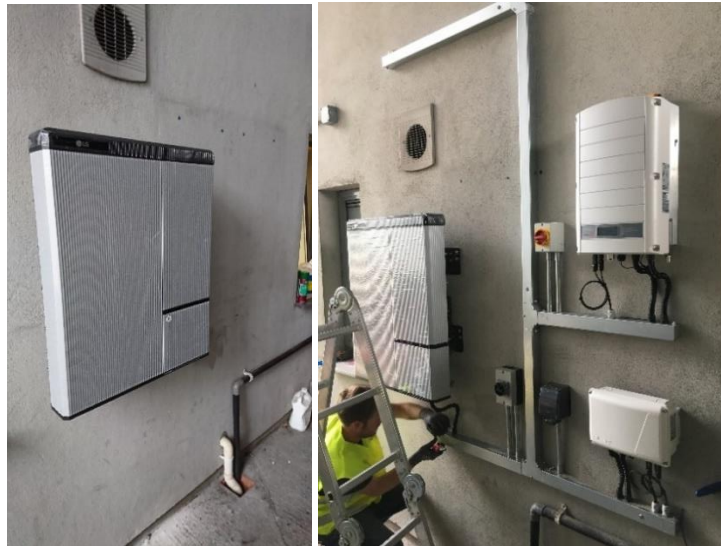
FIGURE 2 - BALLYVOLANE FIRE STATION INSTALLATION
