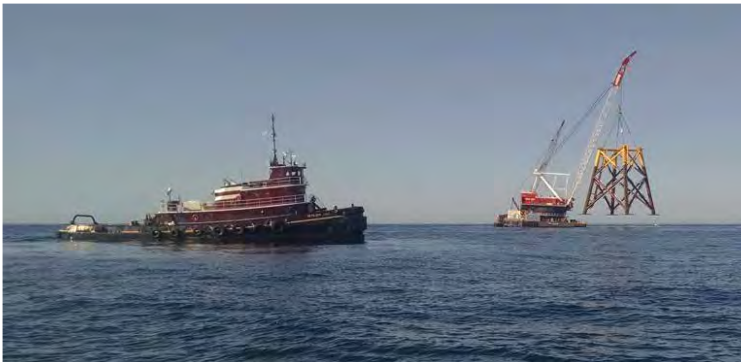
Figure 1. Deepwater Wind's Block Island Wind Farm (Photo credit: Deepwater Wind)
