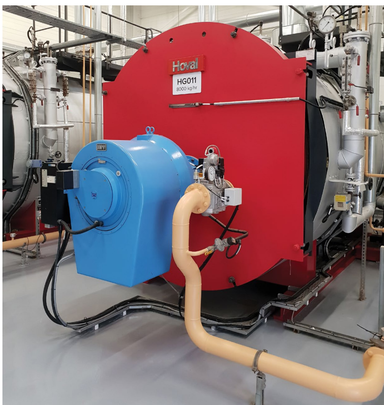
Figure 1: Gilead Steam Generation Boiler
