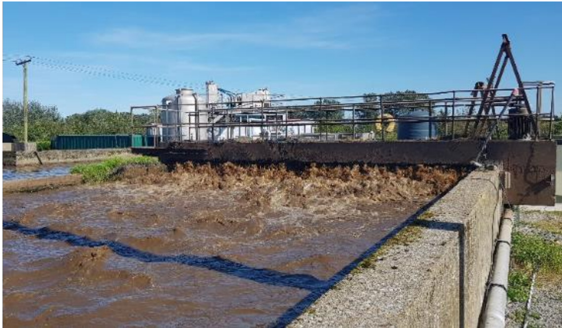
Figure 7: Horizontal brush surface aerator under operating conditions (aerator 1).
