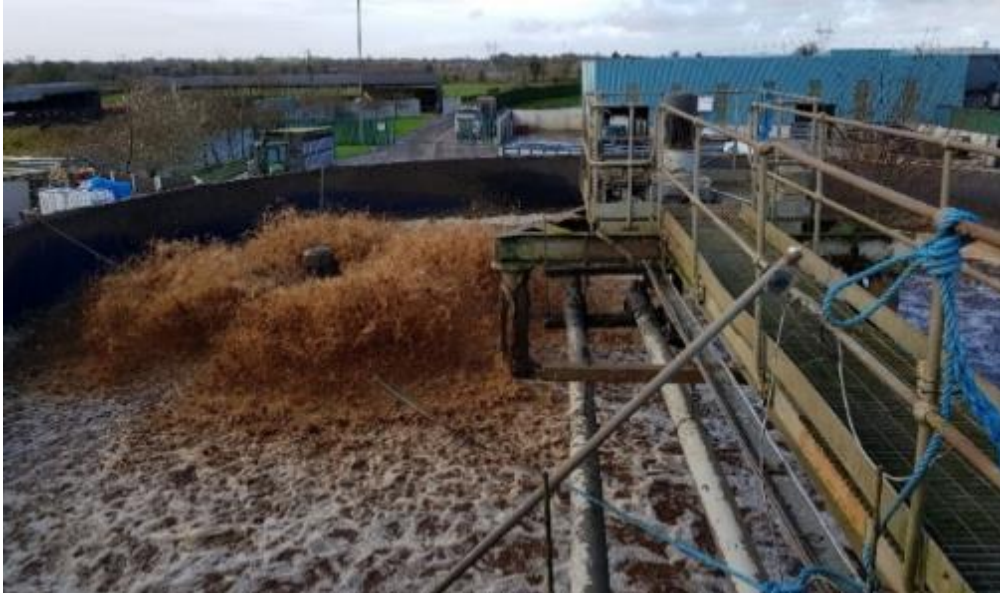
Figure 2: High-Speed Surface Aeration System in Aeration Tank 1
