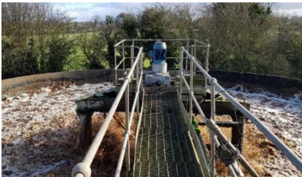
Figure 3: Low-Speed Surface Aeration System in Aeration Tank 2
