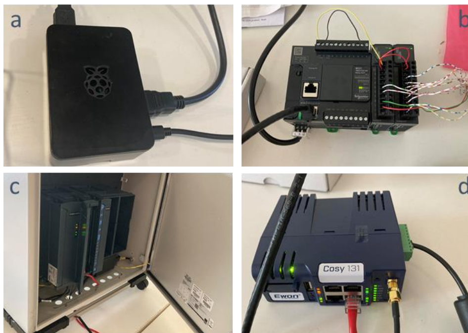
FIGURE 6. A) RASPBERRY PI EMULATING SCADA SYSTEM MODBUS STREAM, B) SCHNEIDER ELECTRIC – PROGRAMMABLE LOGIC CONTROLLER, C) REMOTE TERMINAL UNIT INTERPRETING MEASUREMENTS, D) EWONCOSY 131 – COMMUNICATION TO CLOUD PLATFORM FROM RTU.
