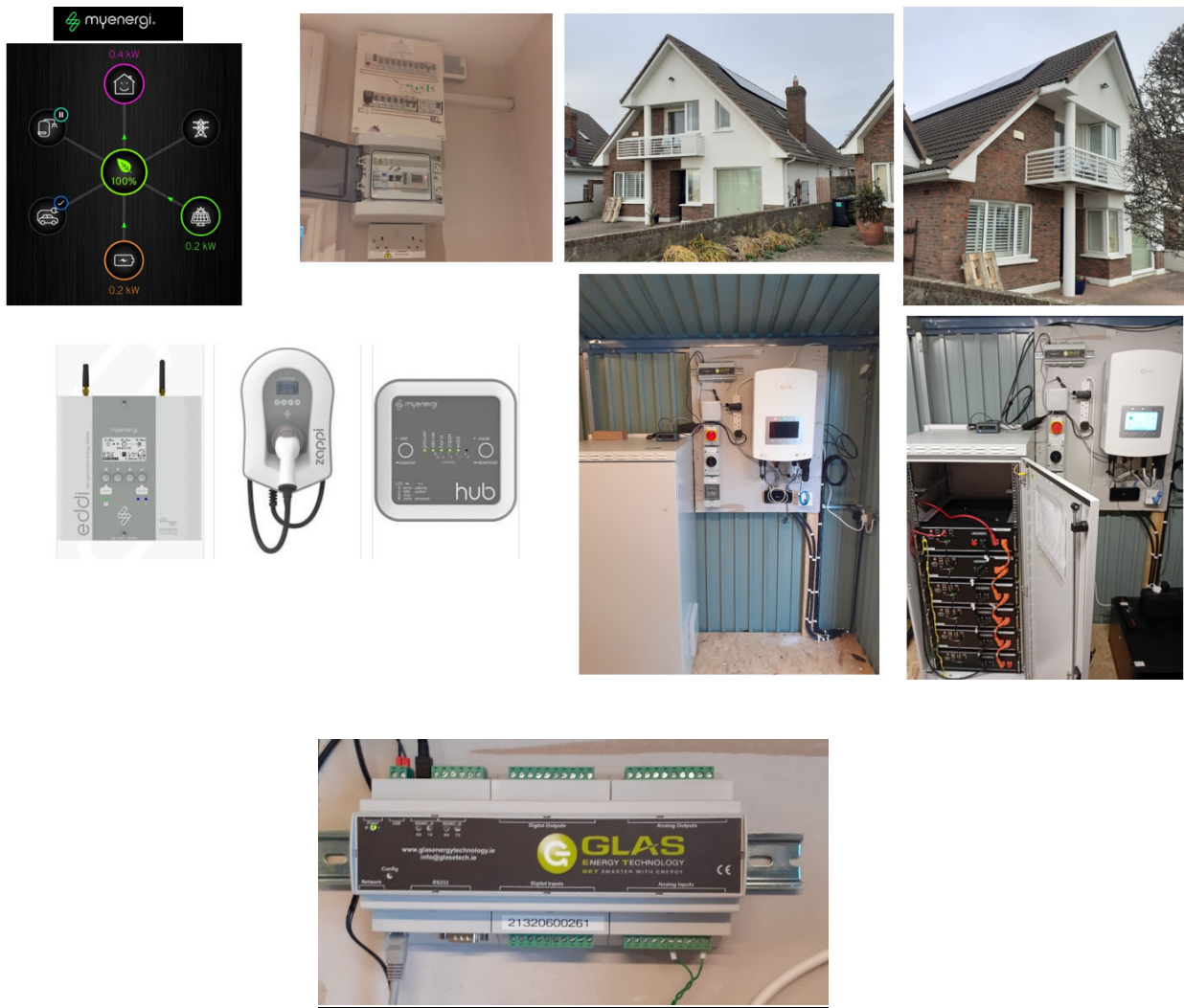
Figure 2 (Pictures of installed devices)
