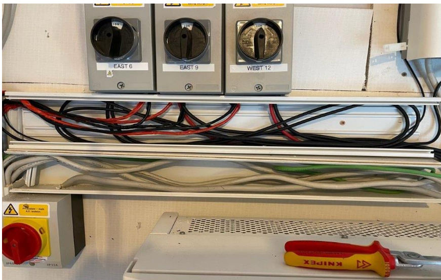
Fig 3: AC/DC run in separate trunking
